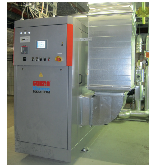
Block- Heiz- Kraft- Werk (BHKW)
